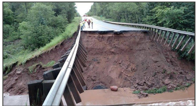
Figure 8 - Road damage after a 10-inch rainstorm in northern Wisconsin in July 2016 (Forest Service photo)
